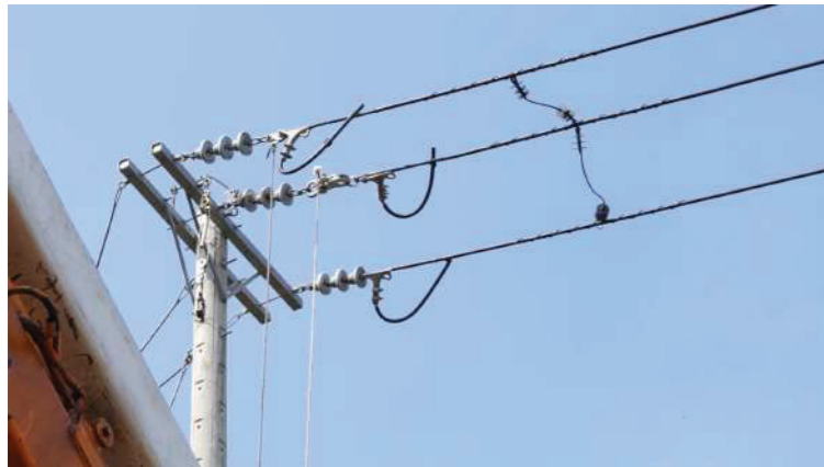
Three-phase power lines with Cable Support Safety Device installed.
