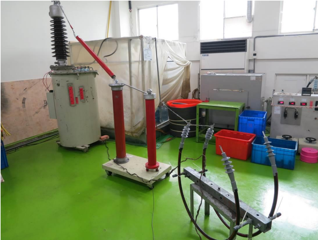
DC Withstand Voltage Test
